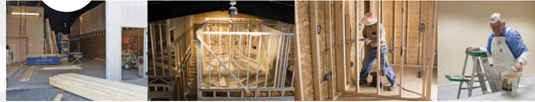
With the help of carpenters, electricians, and painters, the construction of new offices and studios for 3ABN Radio is moving along. We can't wait to move into our new facilities!
